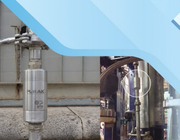
Installation after the water meter
